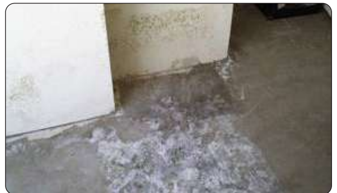
Foto N° 2 Aspergillus en base de terma (Fuente : Building Cleaning Services - California)
